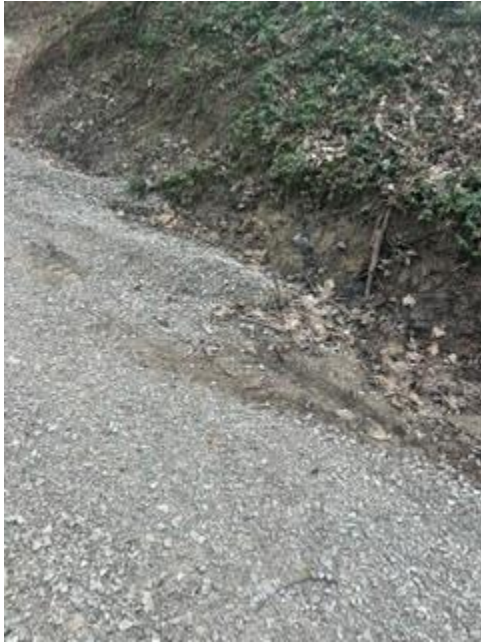
Erosion of swale
