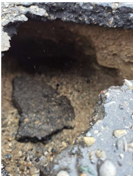
Pavement Settlement & Migrated Granular Documented April 16, 2026 (Site Location - see Figure No. 1)
