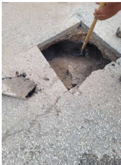
Pavement Settlement & Migrated Granular Documented April 17, 2026 (Site Location - see Figure No. 1)
